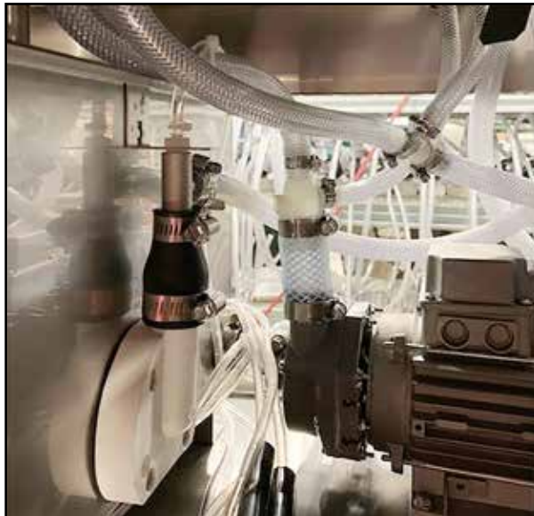
Lower piping configuration beginning with S/N G200325482.
